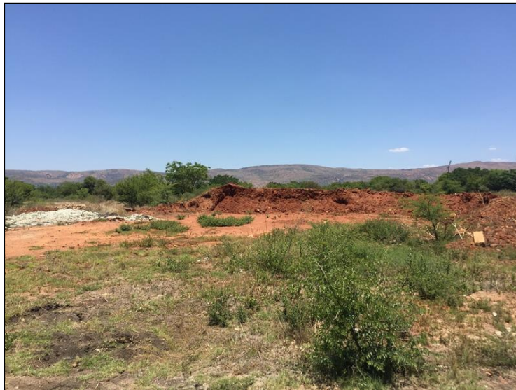
Figure 3-4: View of large excavation and digging in the north of the study area.
