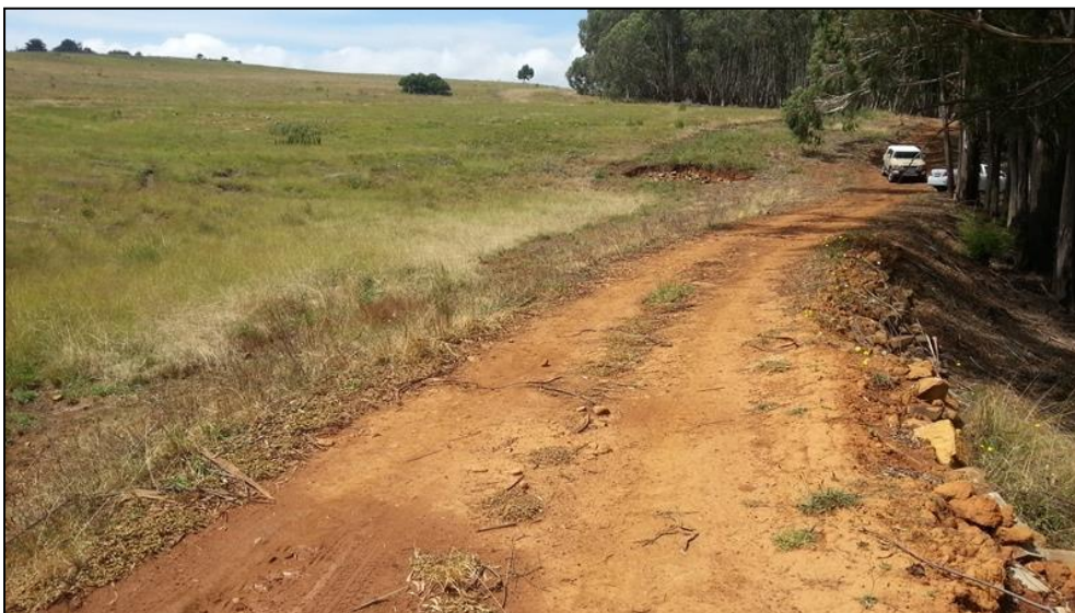
Figure 3-4: View of the study area along the access road where a culvert is proposed.
