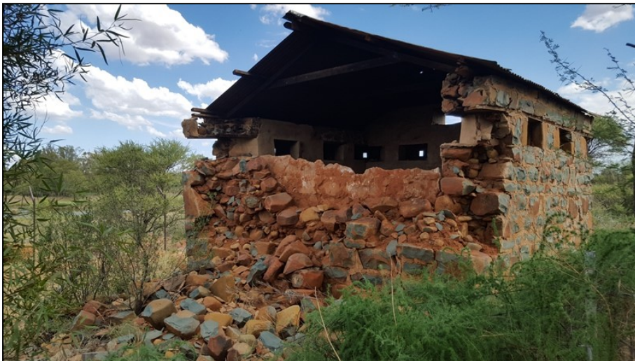
Figure 5-32: View of a side wall loophole above the door of the blockhouse.
