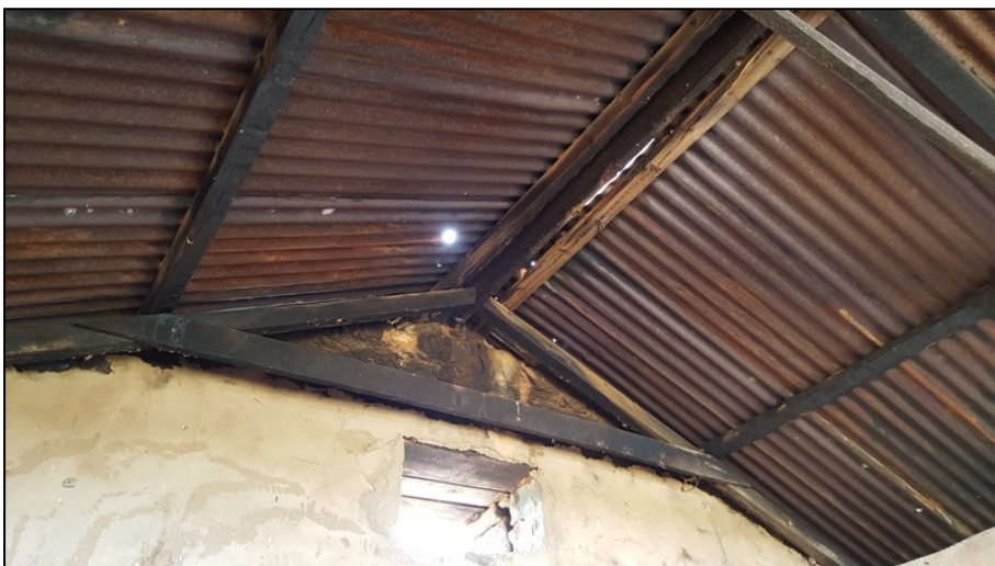
Figure 5-25: View of the interior of the blockhouse; loopholes, porthole and roof structure.
