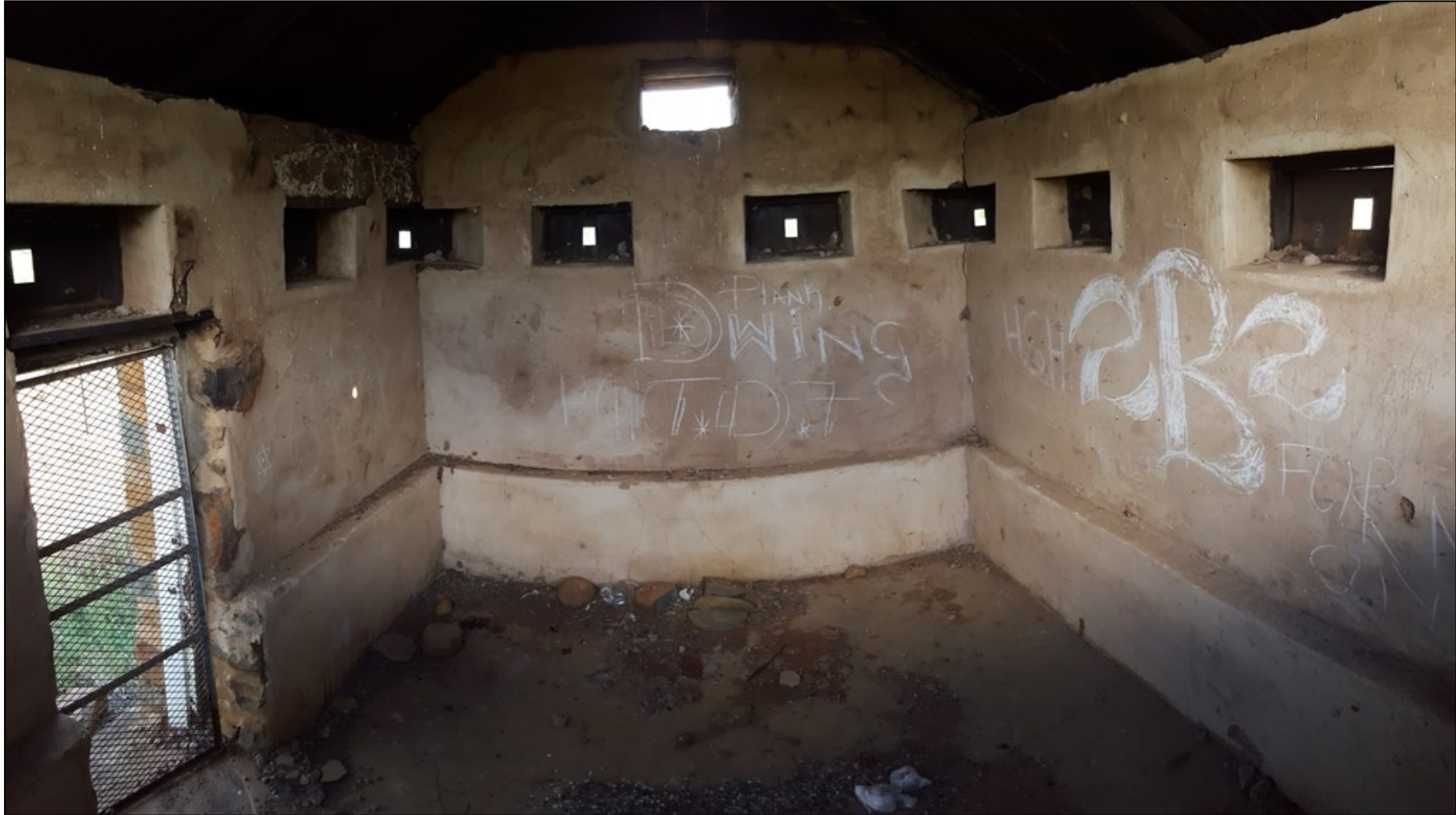
Figure 5-27: View of the southern, western and northern walls in the interior of the blockhouse. Note the firing step along the walls.
