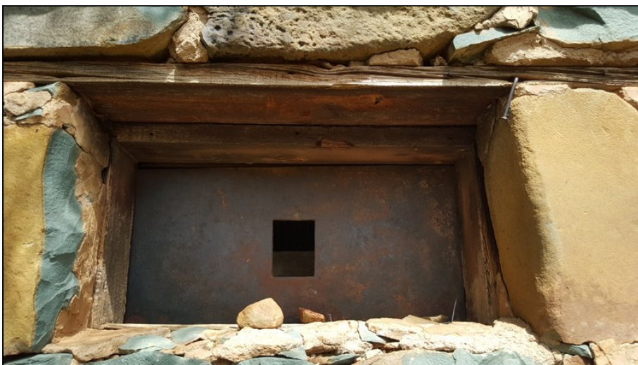
Figure 5-29: Collapsed section of the blockhouse wall revealing stone and red sand mortar construction.
