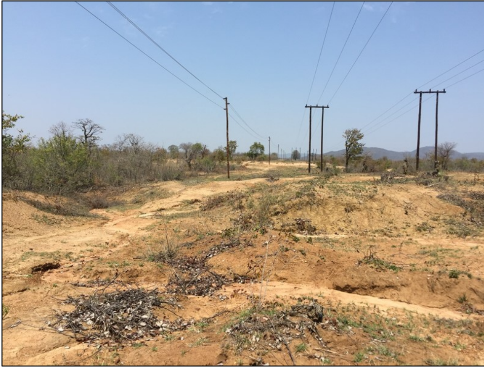
Figure 3-10: View of erosion gullies along power lines forming the eastern boundary of the study area.
