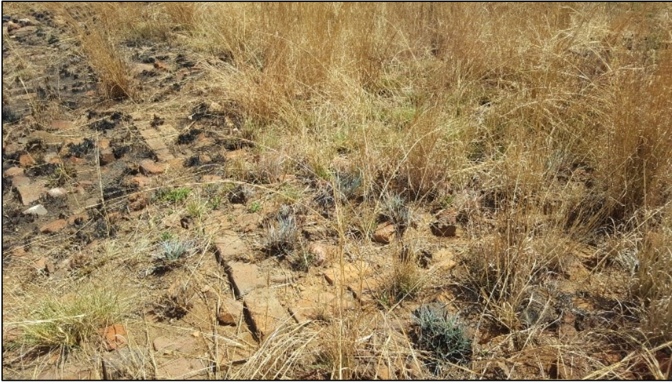
Figure 5-6: Collapsed walling and brick foundations at Site Exigo MDW-HP02.
