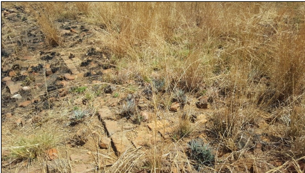
Figure 3-6: Collapsed walling and brick foundations at Site Exigo MDW-HP02 Feature 1.
