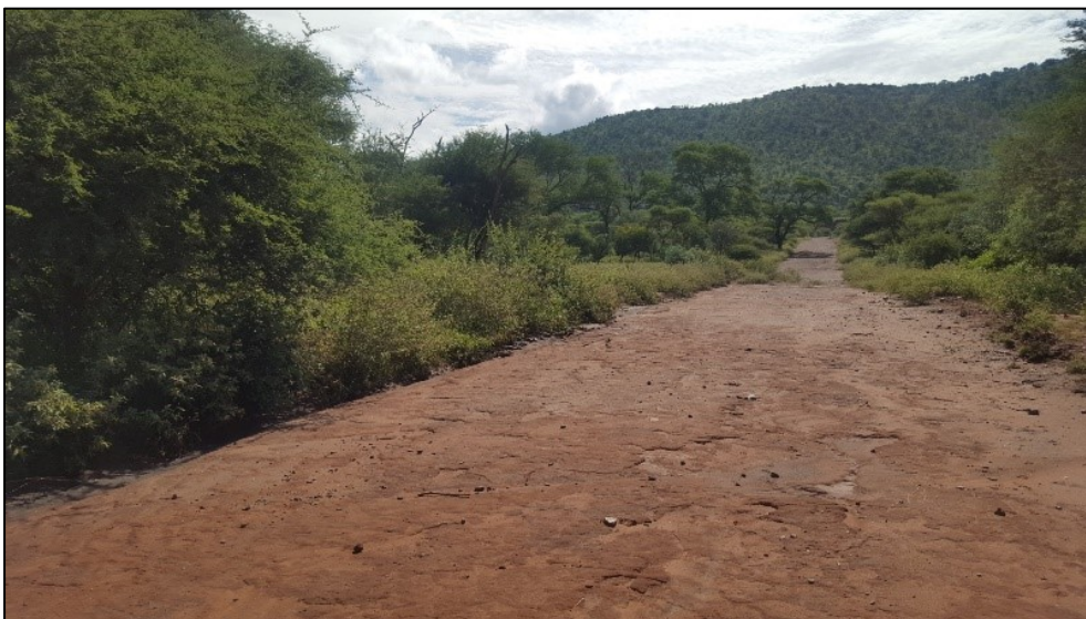
Figure 3-6: View of an access road towards the proposed Q3 borrow pit site.
