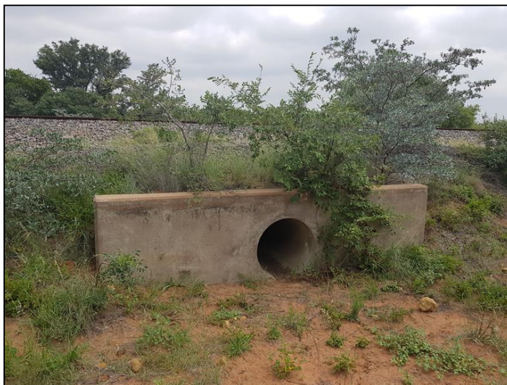
Figure 3-5: View of a culvert which was constructed in 1980 along with the railway line.
