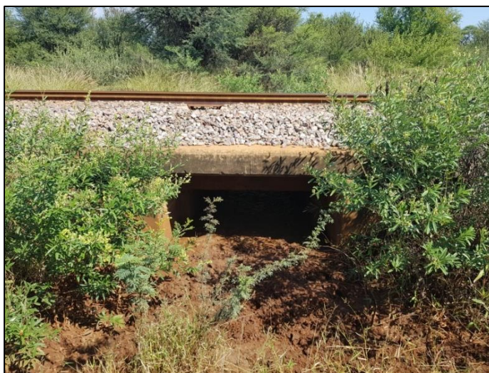
Figure 5-1: View of the box culvert which was constructed before 1948 along with the railway line.
