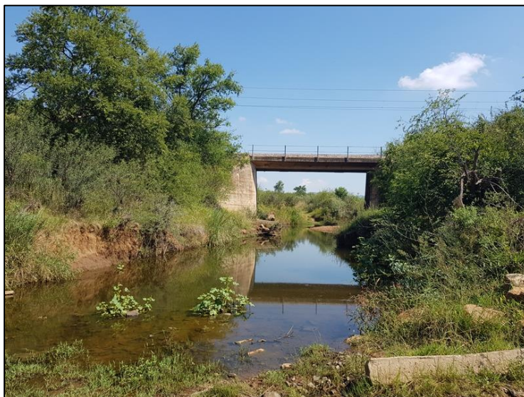
Figure 3-10: View of a bridge over a drainage line north of the proposed railway loop alignment.
