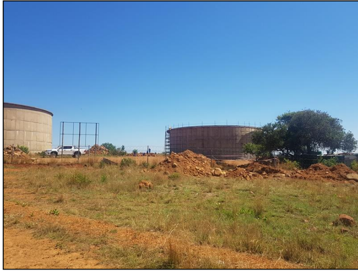
Figure 3-4: View of newly constructed reservoirs along the north-eastern periphery of the study area.
