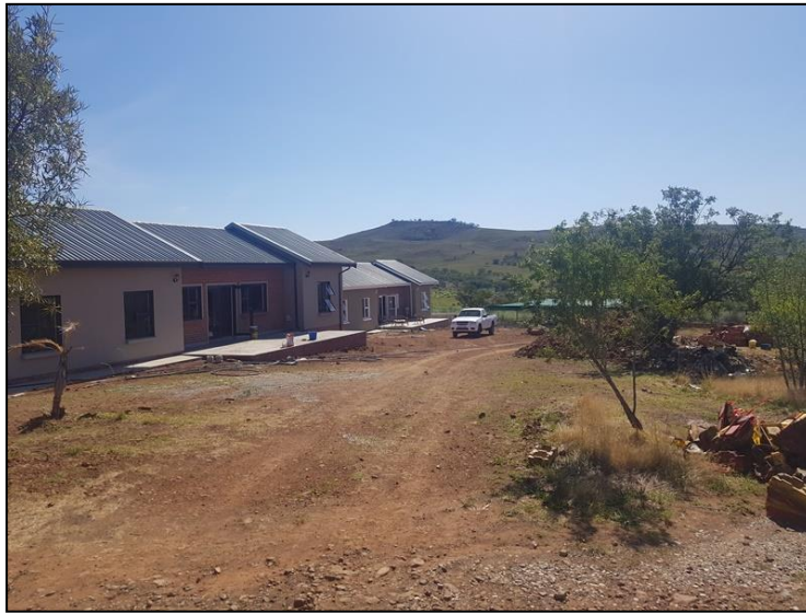
Figure 3-16: View of new buildings for the Door of Hope centre in a southern section of the project area (see Addendum 3).
