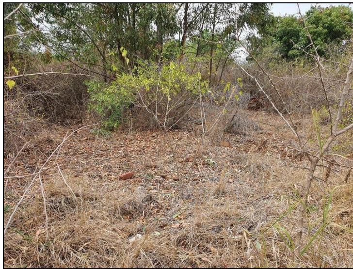
Figure 5-9: View of the poorly preserved foundation structures, presumably of the Beja farmhouse at Site Exigo-BOD-HP01.
