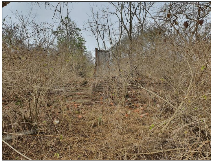
Figure 5-13: View of the poorly preserved building structure at Site Exigo-BOD-HP03.
