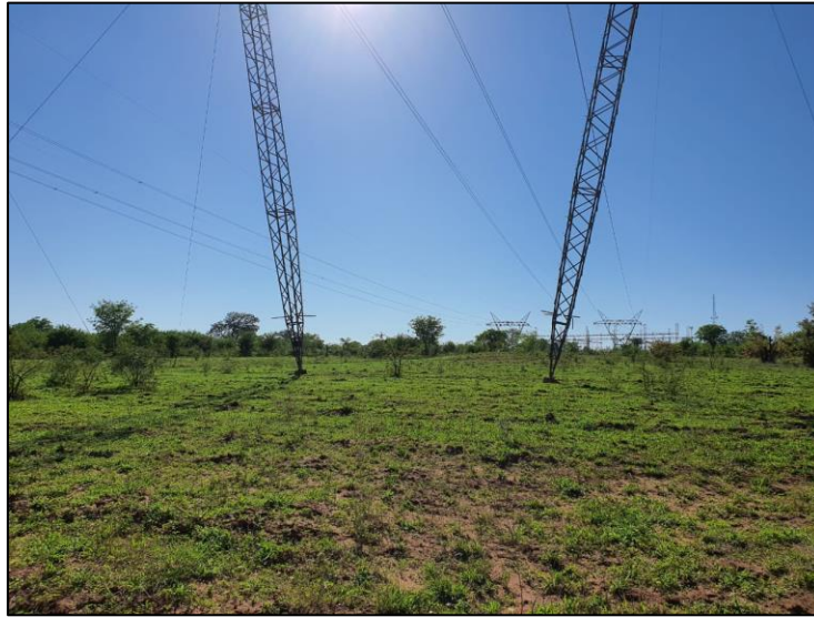
Figure 3-8: View of the current Eskom Power line along the project area corridor.
