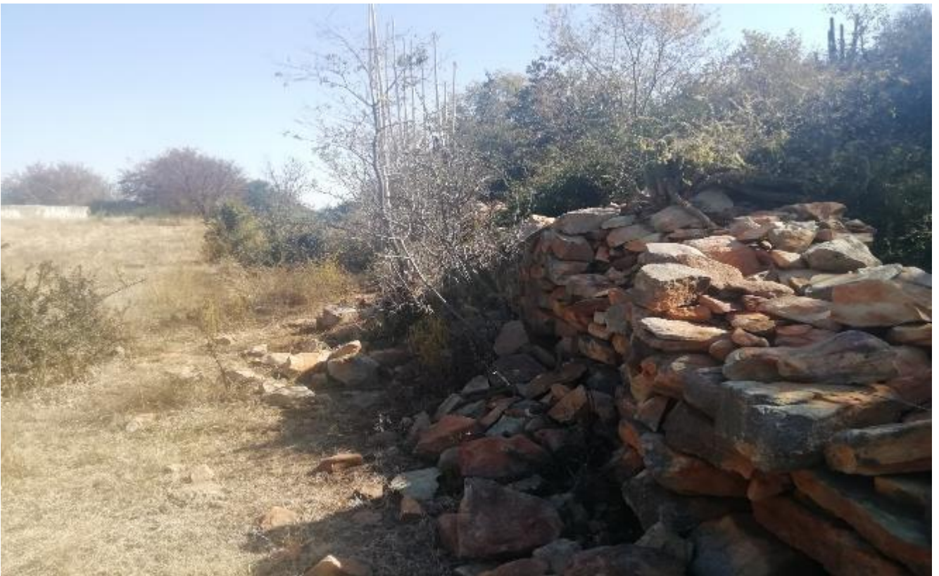
Plate 27: showing collapsing stone wall on northern section of the site.
