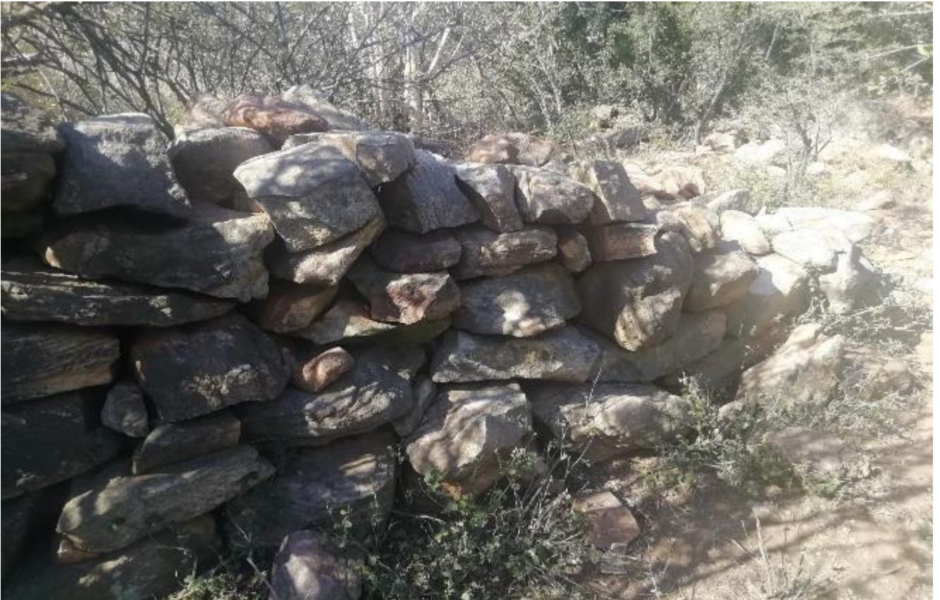
Plate 28: showing bulging stone wall on the site.
