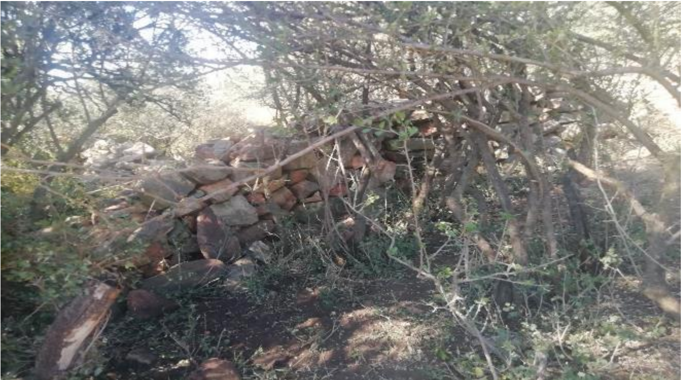
Plate 26: showing overgrown vegetation on the surviving stone walls..
