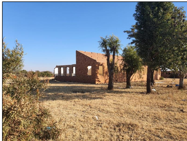
Figure 3-6: View of a partially dismantled brick building associated with the shooting range.
