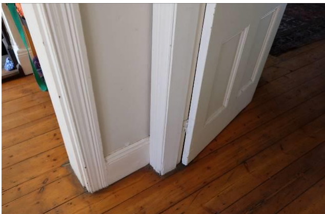
Fig. 70_Original wooden skirtings and door frames in most of the rooms still in good condition (Source: tsica heritage consultants, 22.09.2020)
