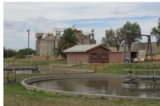
Primary settling tanks
