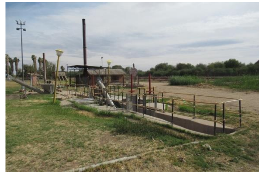
Inlet pump station
