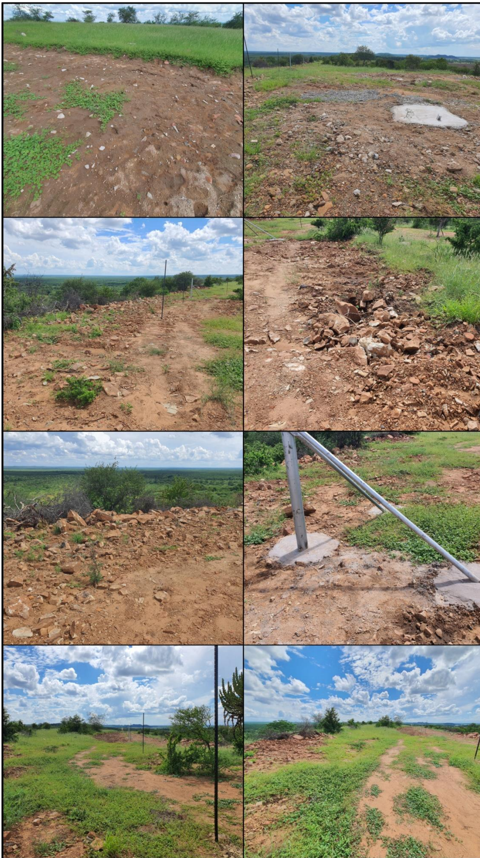
Figure 5-34: A selection of images indicating extensive damage to Site EXIGO-BFD-S3.
