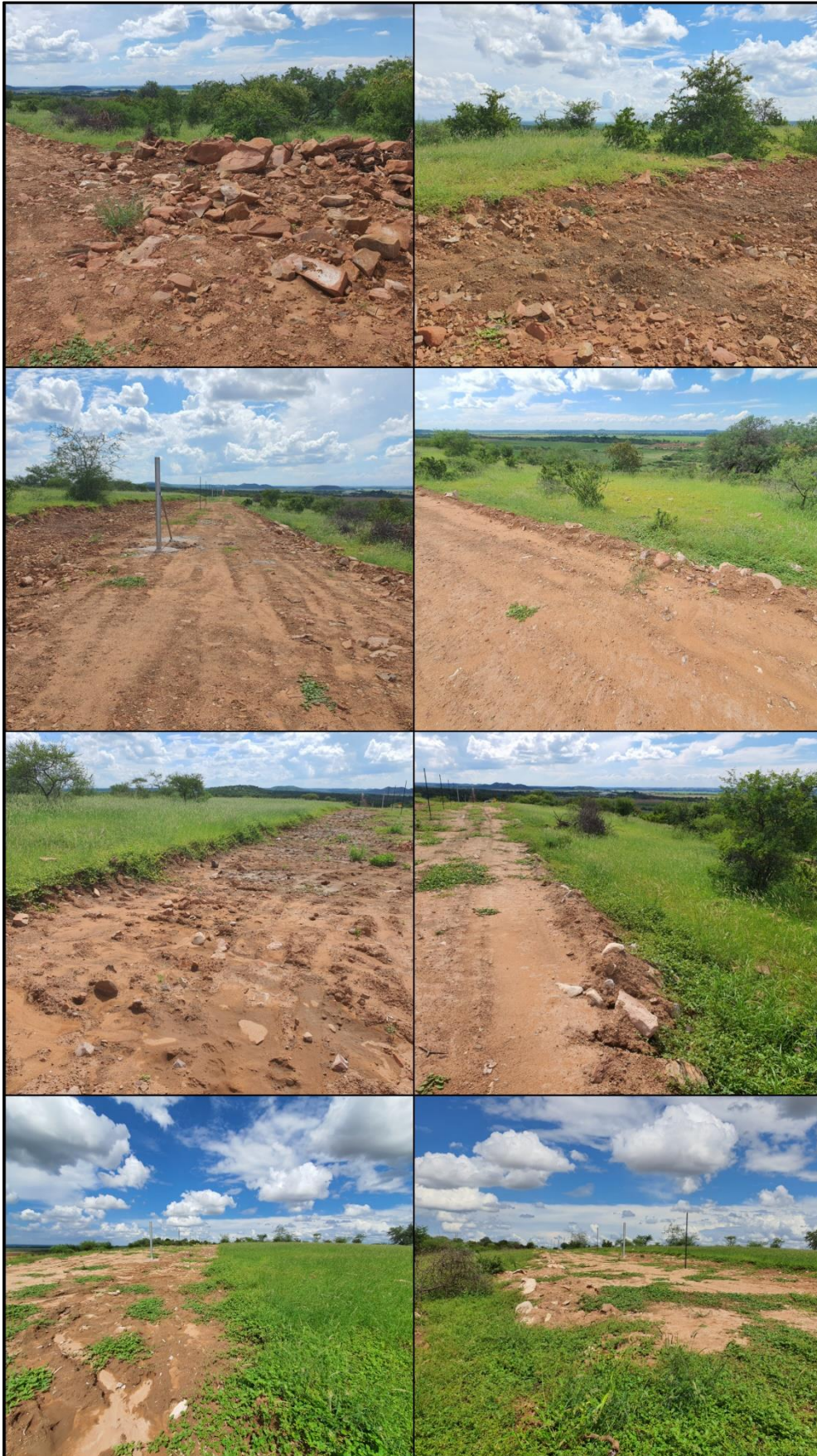
Figure 5-33: A selection of images indicating extensive damage to Site EXIGO-BFD-S3.
