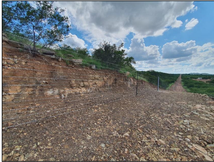
Figure 3-8: View of excavated surfaces to as part of the fence and service road construction.
