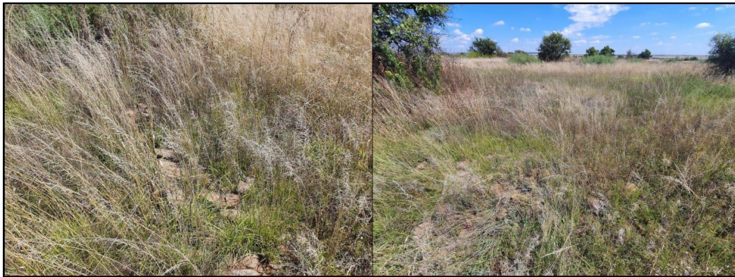
Figure 5-9: View of densely overgrown collapsed stone wall foundations at Site EXIGO-VSP-IA01.
