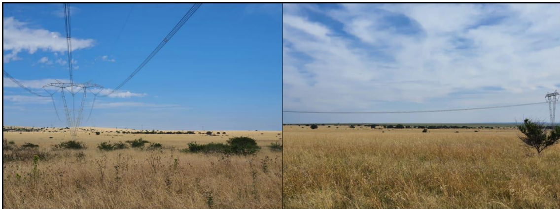
Figure 3-1: View of general surroundings and grasslands in the project area along the exiting ESKOM Powerline servitude.
