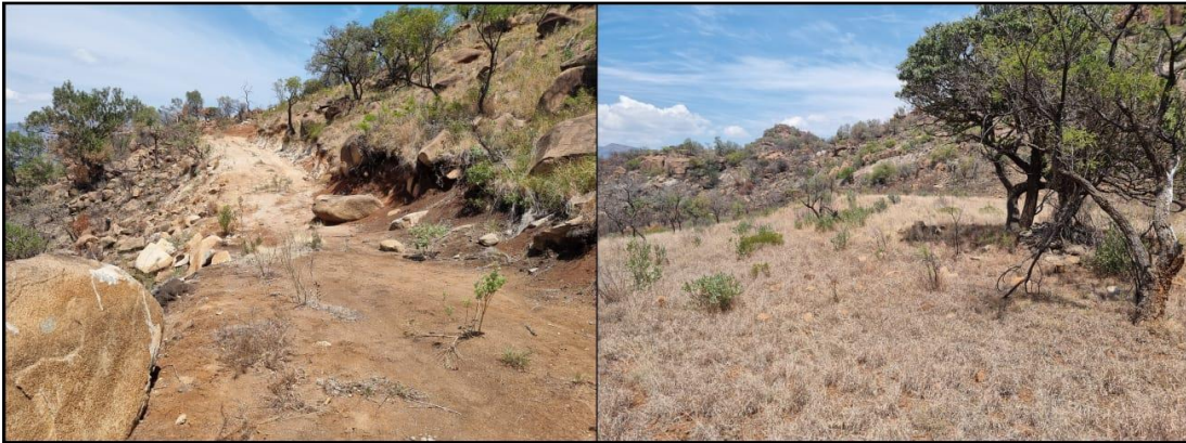
Figure 4-2: View of an eroded access road and general surroundings in the project area.
