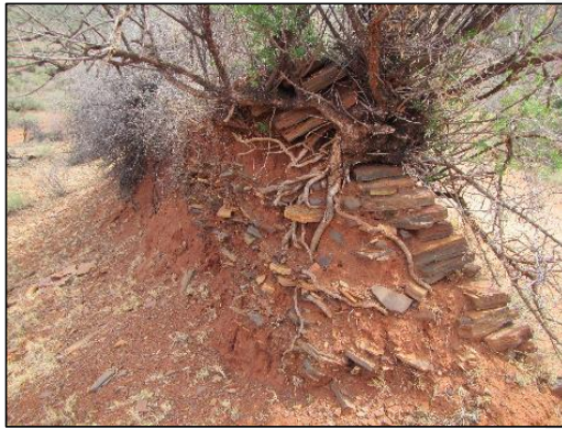
Figure 35: Remains of anti-erosion walls
