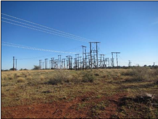
Figure 1: View of the Mothibistad Substation.
