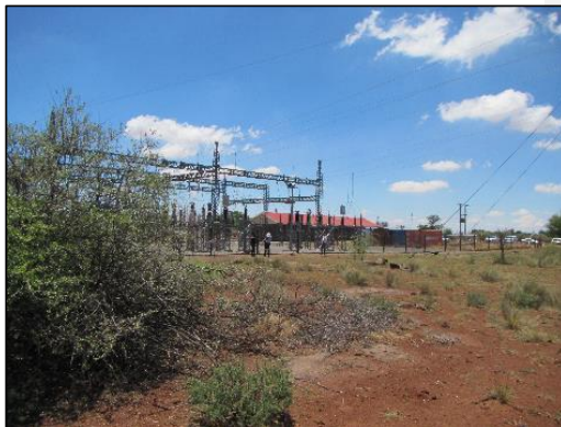
Figure 4: View of the Moffat Substation on the western side of Kuruman.
