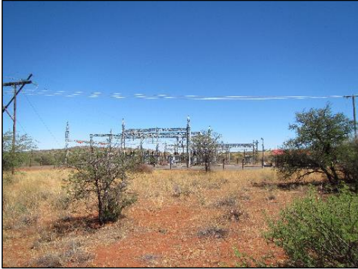
Figure 7: View of the Valley Substation.
