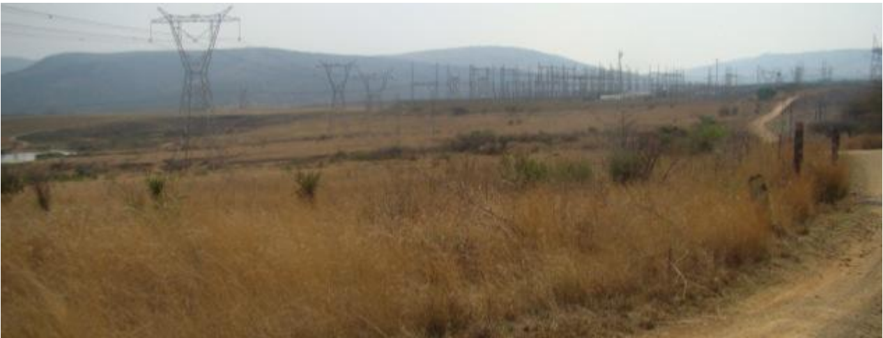
Plate 1: View of Umfolozi Substation where the proposed powerline will T-off.
