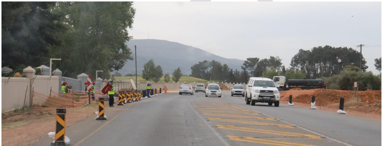
Figure 20: Site photograph illustrating the character of portions of the R301 nearer to Paarl (Smit, 2022)
