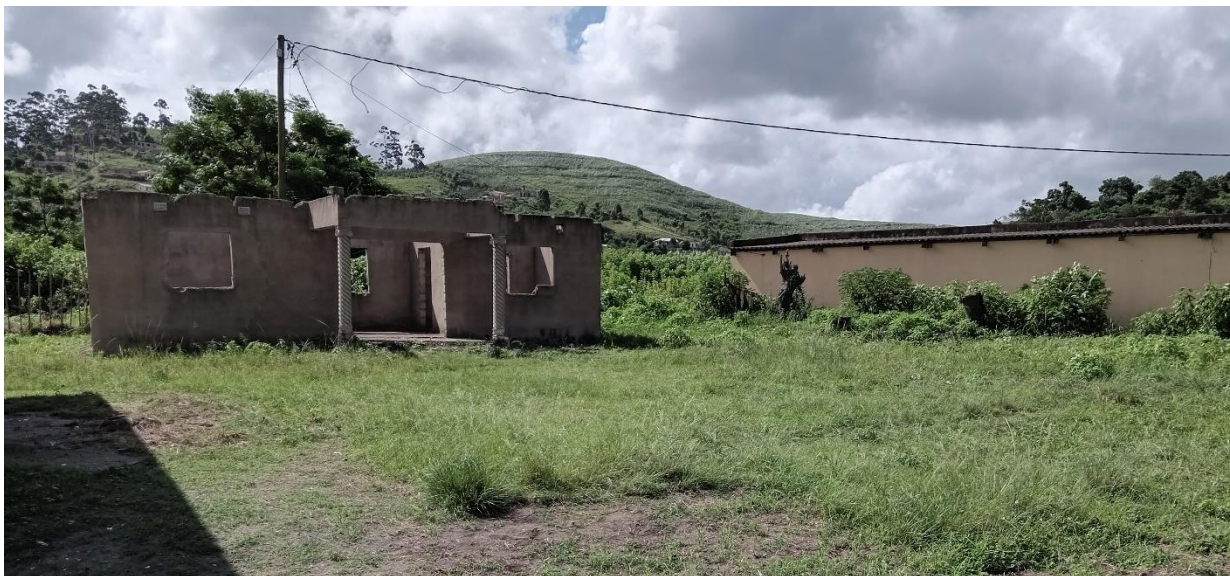
Figure 20: View of the abandoned, partially constructed recent house
