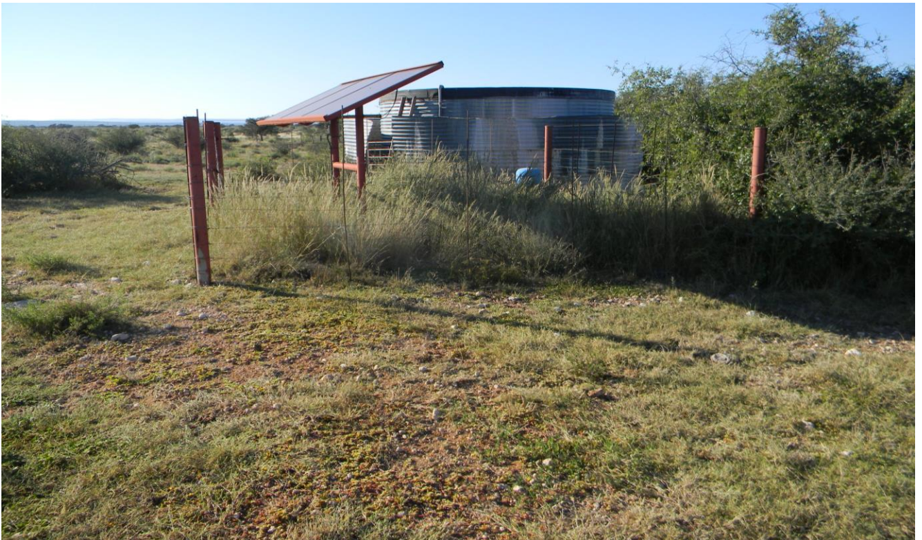
Plate 4: Photo 4: View of water pump and reservoir at the proposed prospecting site (Photograph © by Author 2020)
