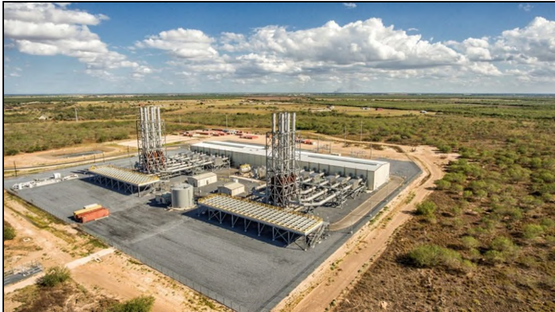
Figure 4: South Texas Electric Cooperative's 225MW Red Gate Plant with reciprocating engines. Photo: South Texas Electric Coop., Inc.
