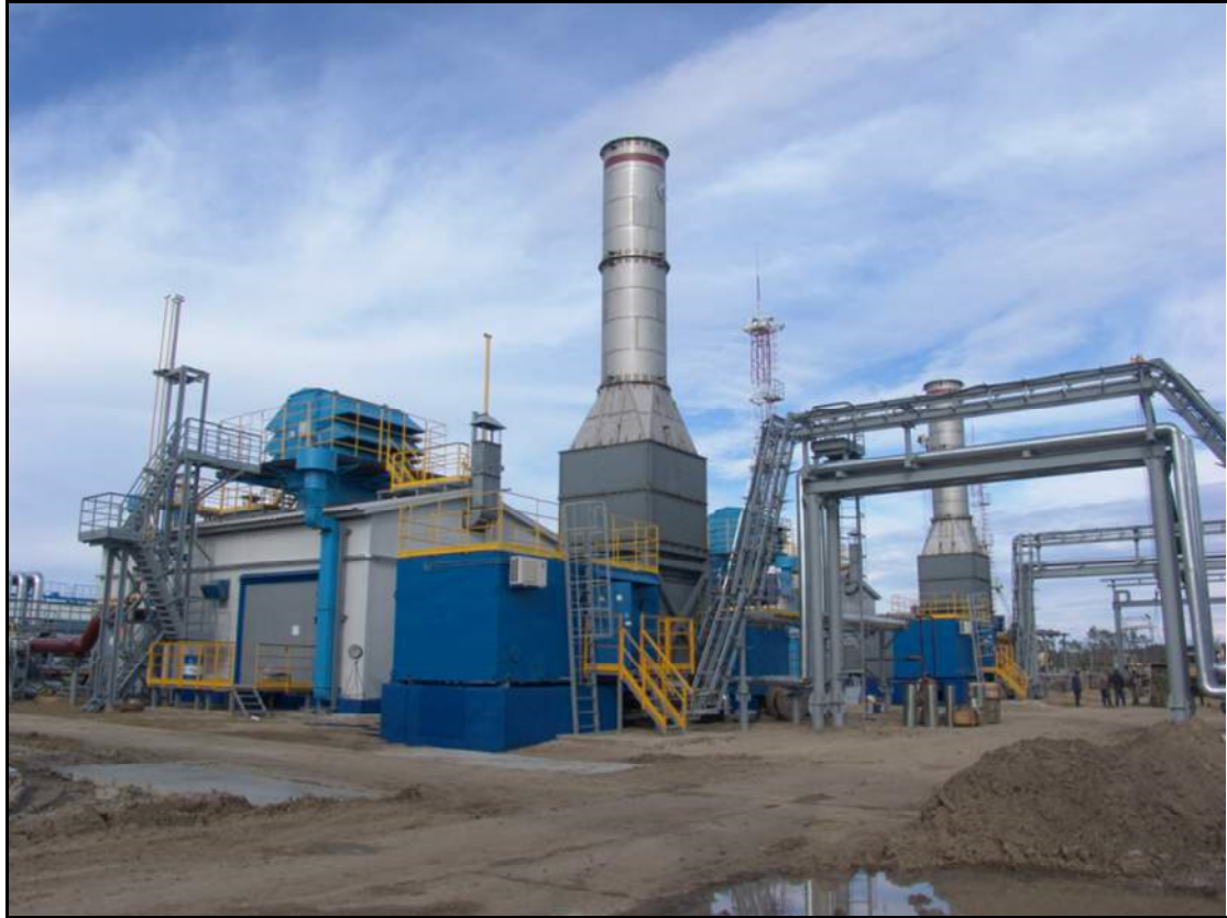
Figure 5: Example of a gas turbine power plant. Photo credit: Unknown.
