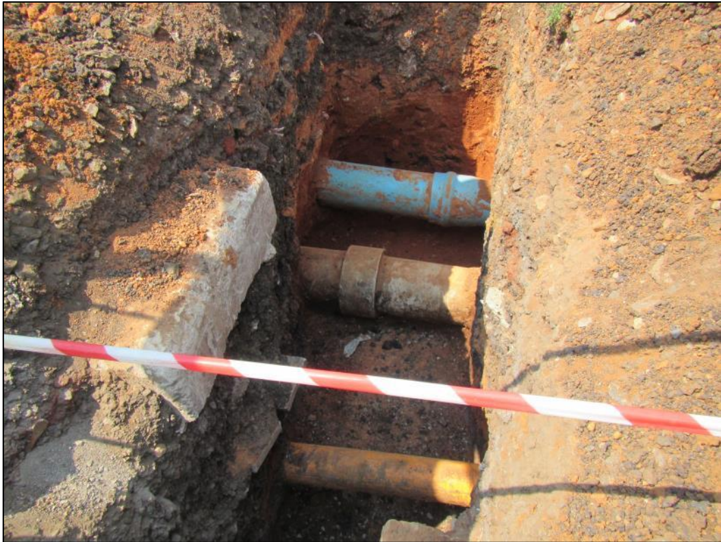
Figure 10 – View of another test pit confirming existing services, located at the point where the railway line and proposed pipeline cross Martinus Rass Avenue.
