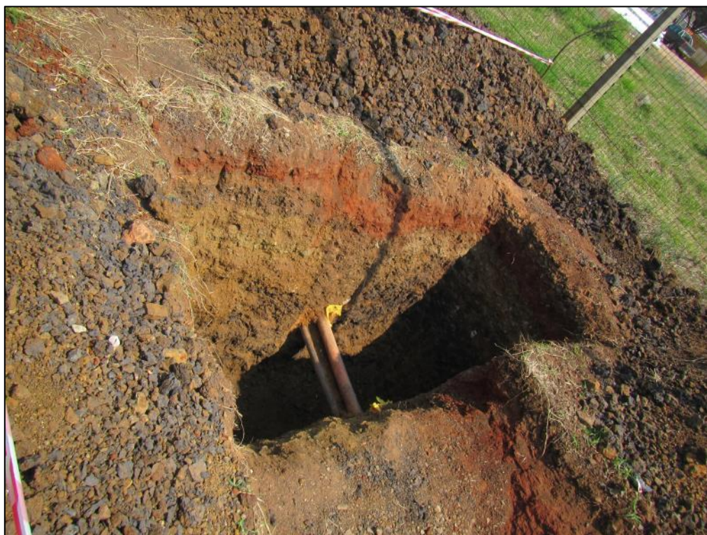
Figure 9 – View of test pit dug to confirm existing pipeline services, located at the entry point to the SAB premises
