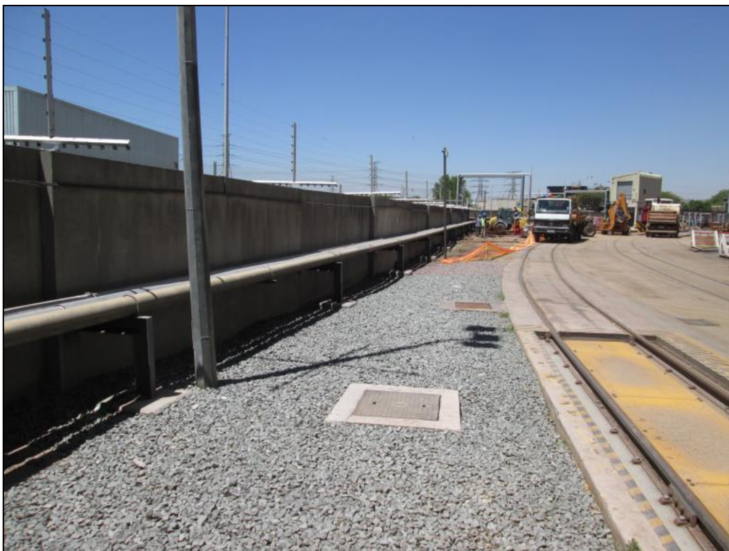
Figure 5 – View showing the existing Sasol gas pipeline within the built-up area of the Rosslyn Brewery. The new pipeline will run on a similar route alongside the existing pipeline.
