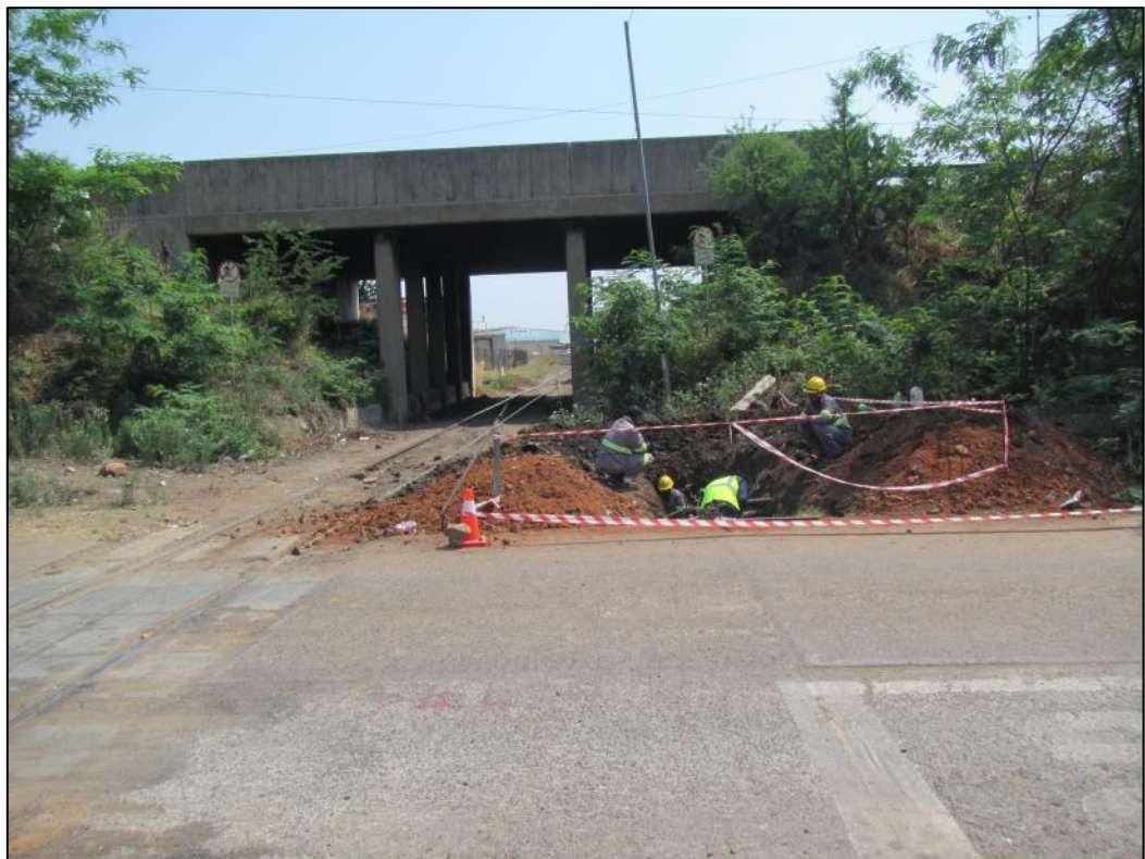
Figure 11 – View where the pipeline route and railway line pass under the R566 road (and cross Marthinus Rass Avenue), showing the test pit location
