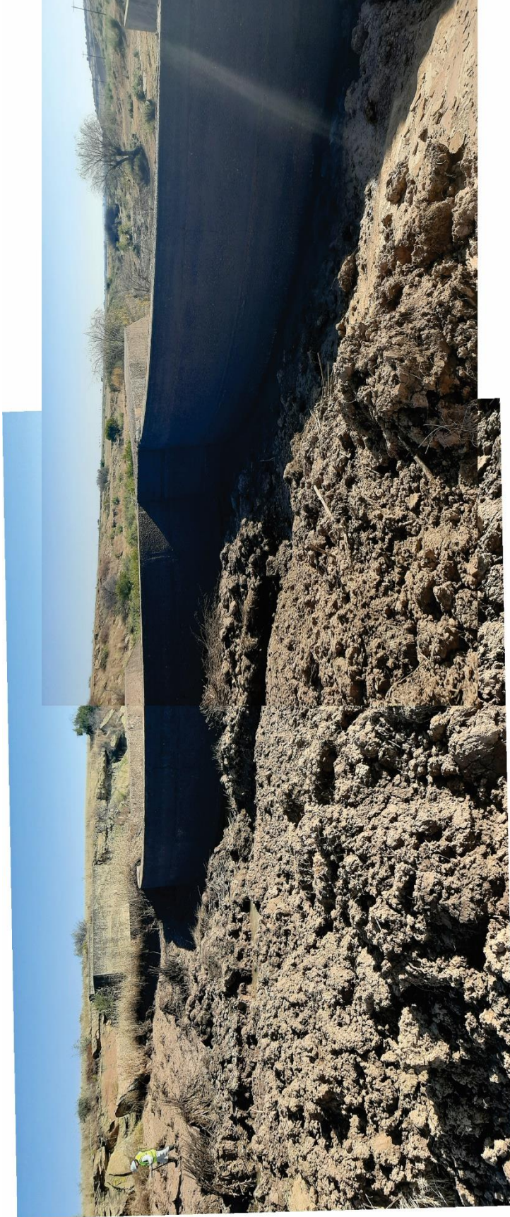
Figure 15. Concrete weir at the northern boundary of the study area, looking west.
