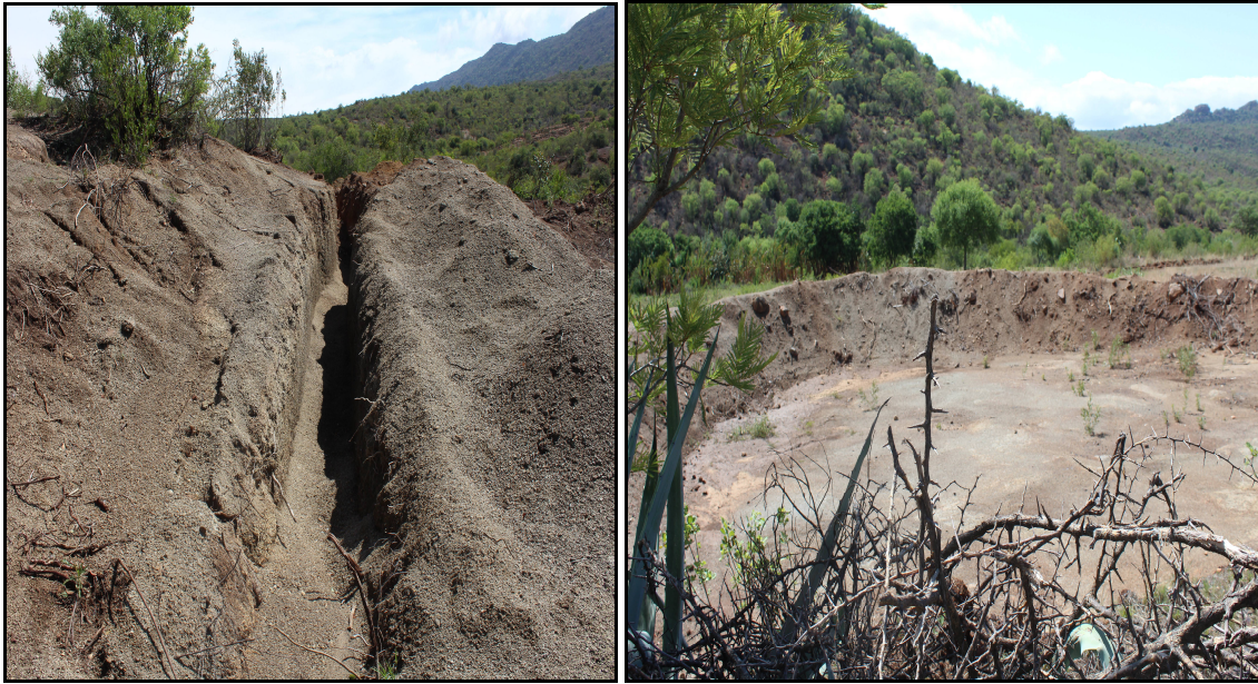
Figure 5: Recently excavated trench earmarked to channel water from the Shakwaneng River to water the nearby garden. The second photo shows an earth dam constructed to store water inside a garden.
