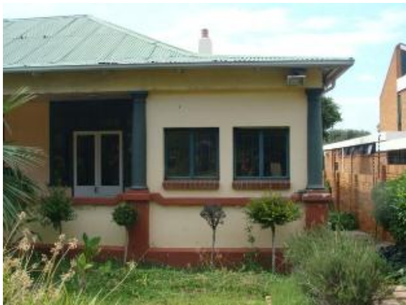
Figure 28: View of a section of the northern part of the house. Schoeman street view.
