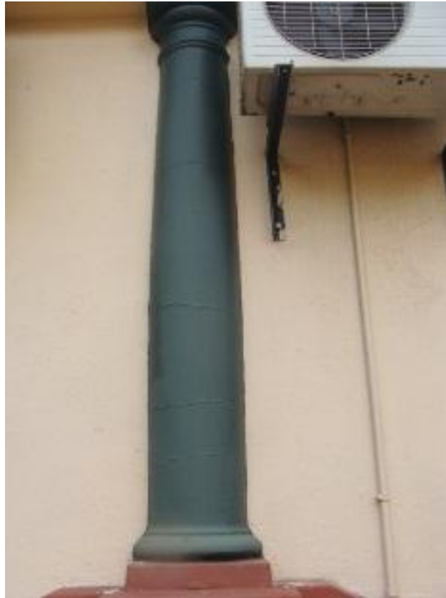
Figure 29: View of a section of the west wall. Original pillars (as per northern view) have been enclosed at some stage.
