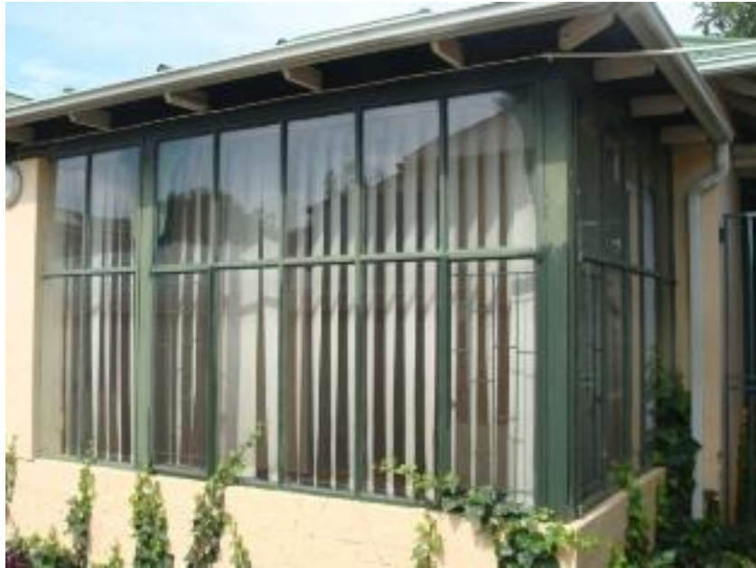
Figure 27: Sun room. This might have been added at some stage, but was not a recent addition.
