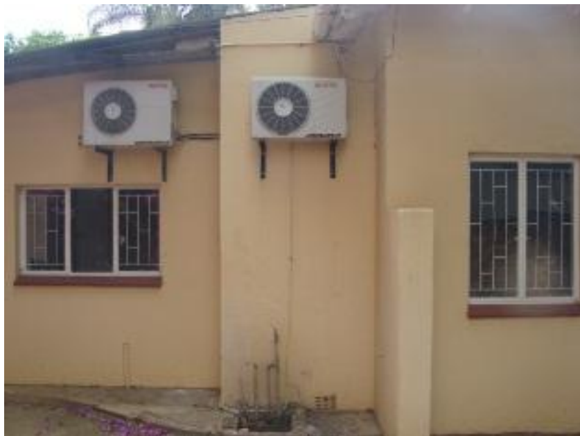
Figure 14: View of western side of house. Most of this are new additions.
