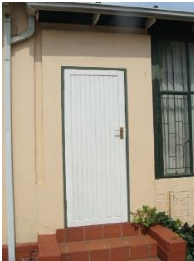
Figure 26: Another view of the east wall. The section left of the door is the added part.
