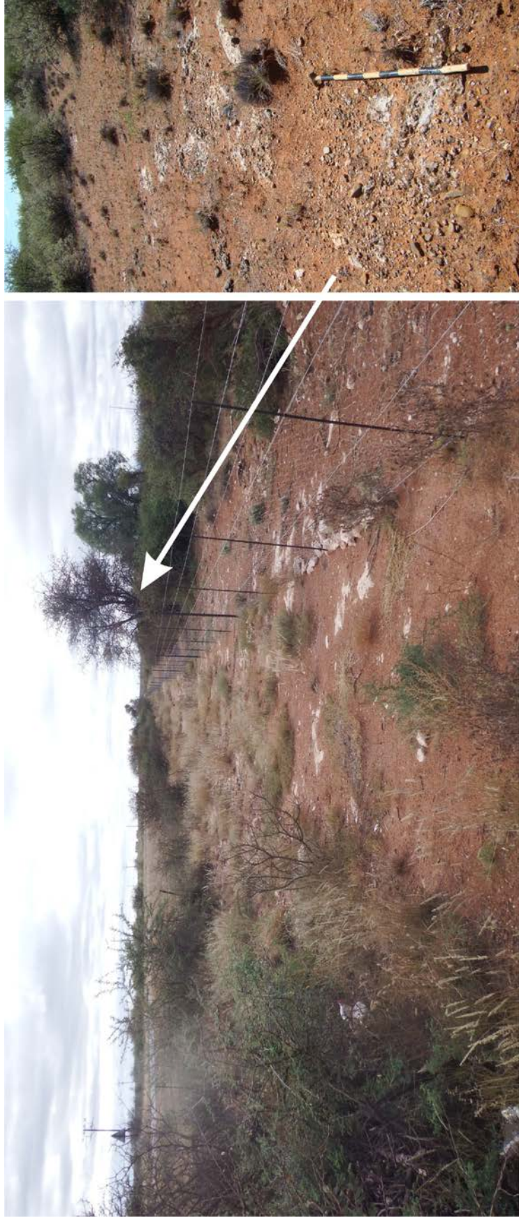
Figure 5. Section A - B, looking north. The 7.2 km long, 900 Ø pipe line is located next to an existing pipe line that follows R325 road about 12 m to the right of the tar surface.
