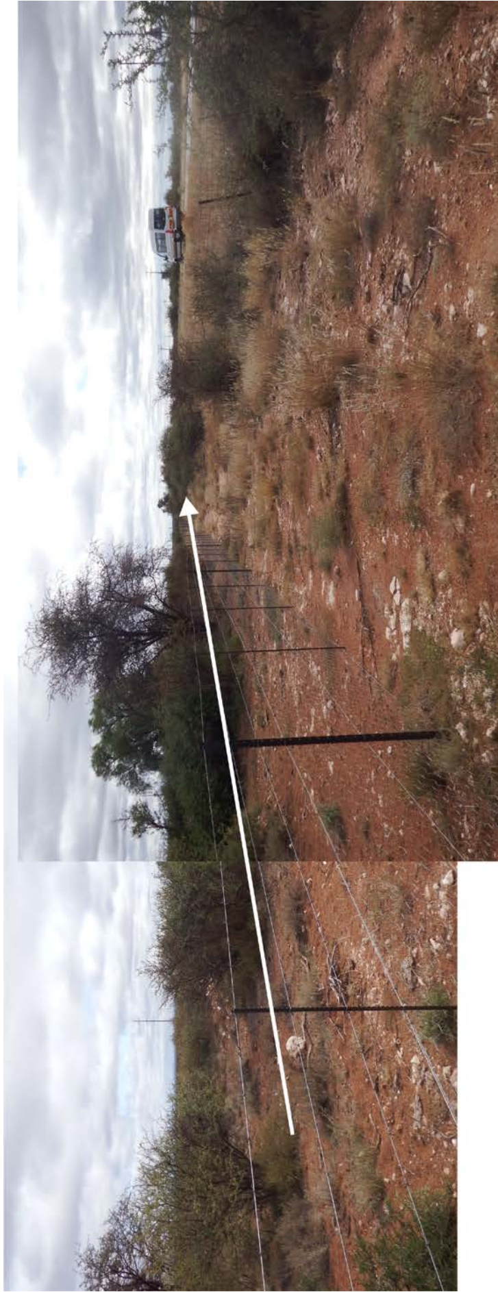
Figure 10. The preferred pipeline deviation will follow the R380 along the left side of the tar surface going north.
