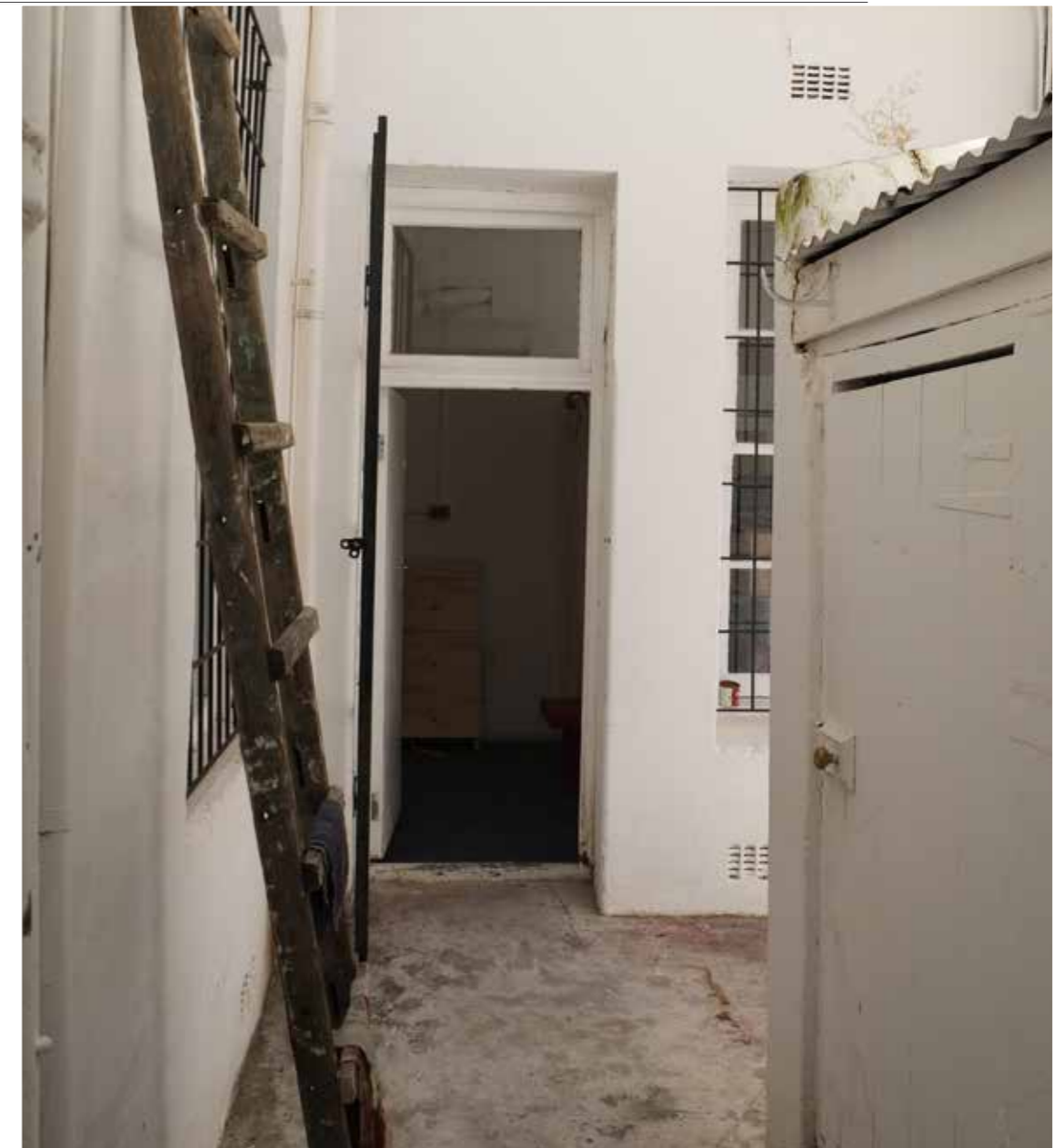
Figure 42. View of rear door from north extension to courtyard, with outbuilding (left). Window (just visible) rebated to internal wall shows the influence of British construction techniques suggesting that the north extension is a later addition
