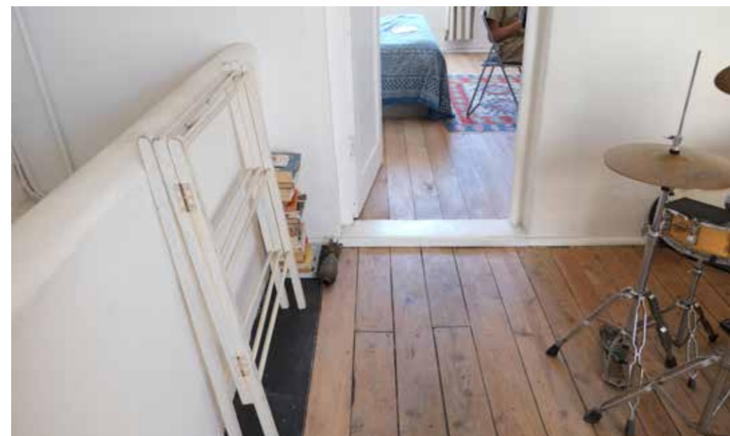
Figure 22. First floor changes to layout (exterior wall removed, slab extended over passage (concrete surface), internal wall added over timber floor)
