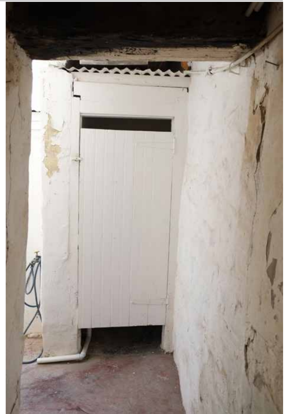
Figure 38. Beneath the stairs and passageway looking to rear ground floor outbuilding (W/C) south
