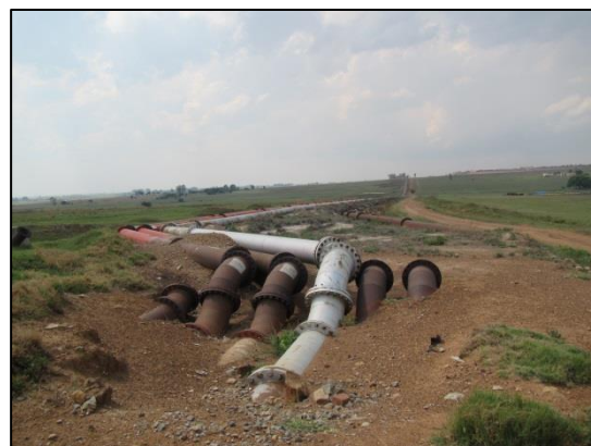
Figure 7 – View of Rooikraal pipeline where it emerges from underground at a point along
