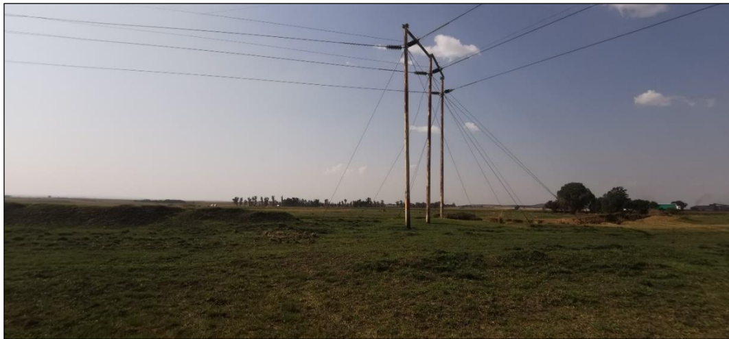
Figure 28 - General view of powerlines located in the AMSA – 3 area.
