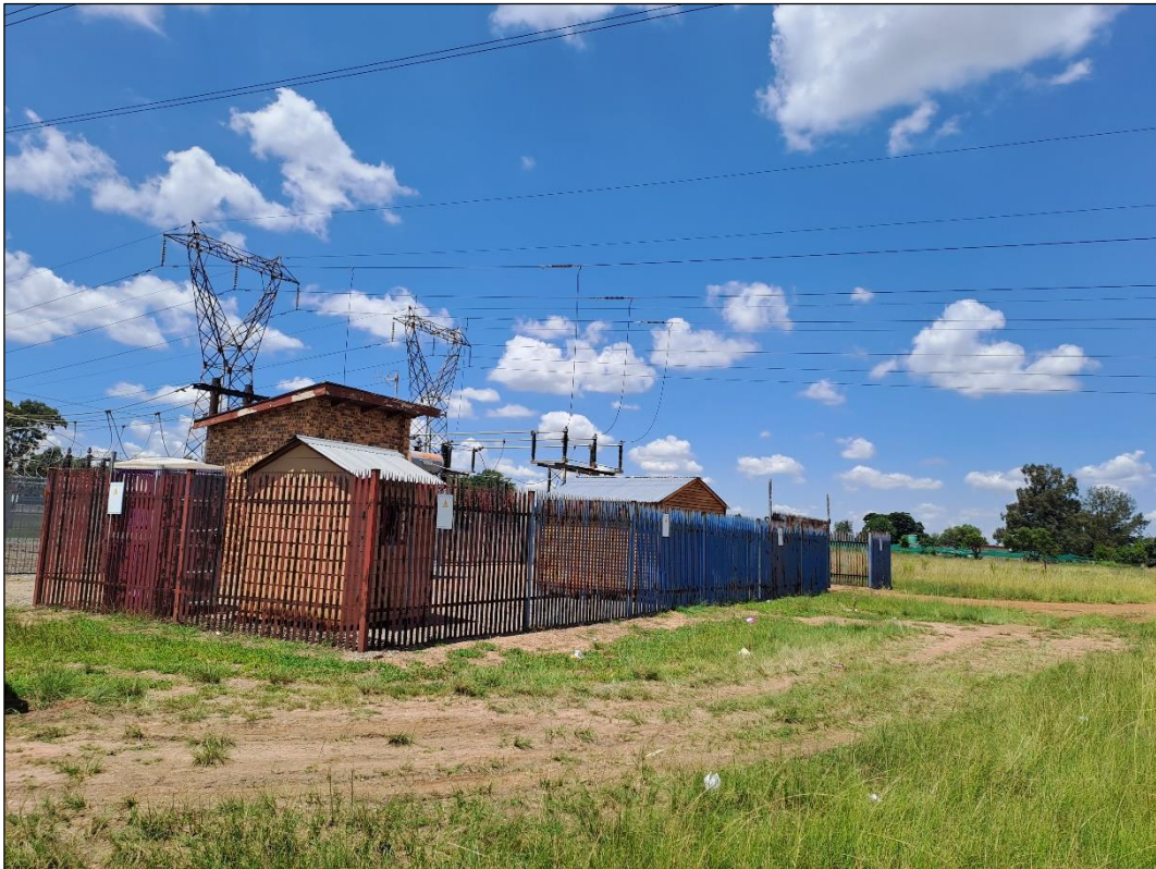
Figure 39 - Sub-station located within the AMSA – 5 area.
