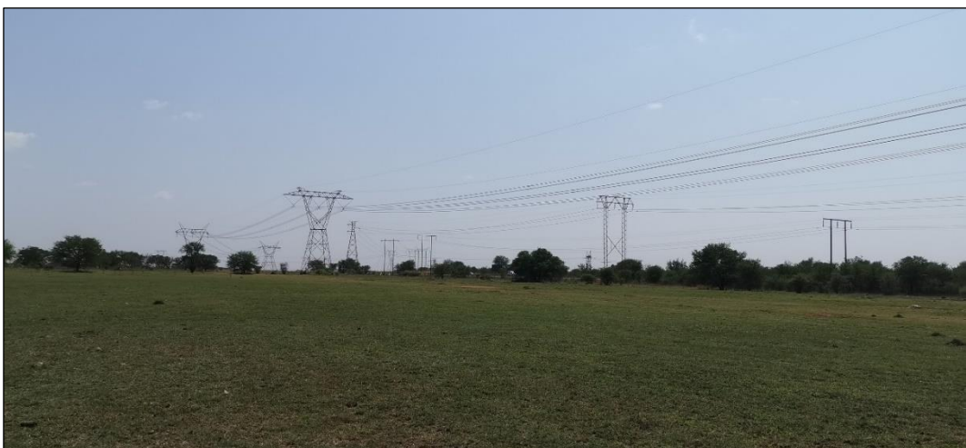
Figure 18 - General view of powerlines located in the AMSA – 1 area.
