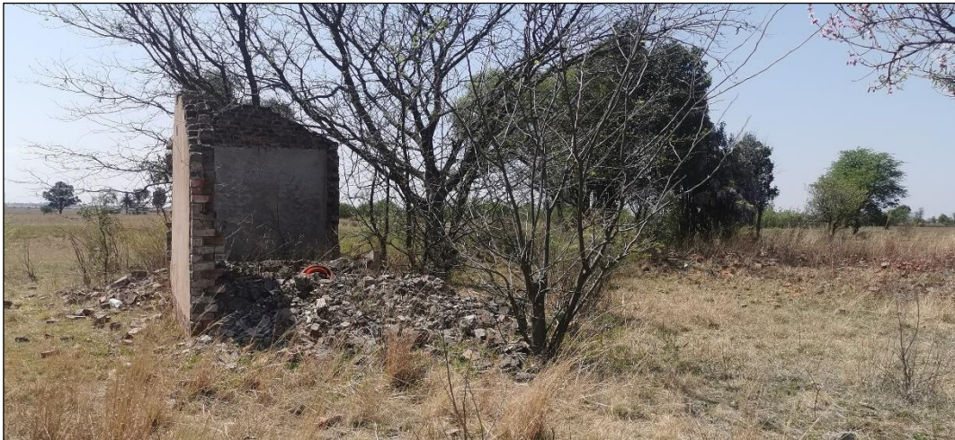
Figure 55 - Site VDB06 which is the remains of a broken-down structure. The building consists of bricks and concrete.
