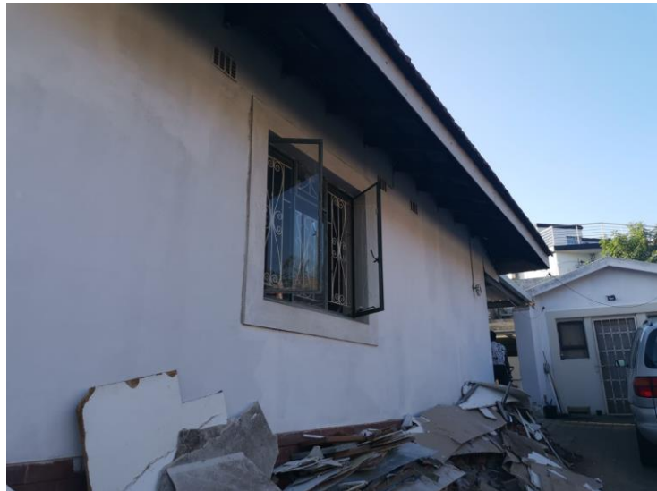
Image 14. Image of the Side East Elevation and South elevation of the outbuilding (First Site Visit)
