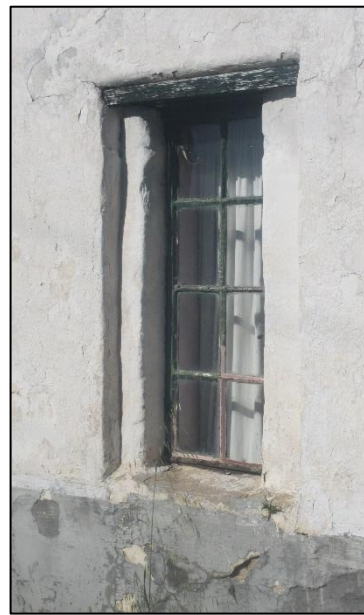
Close up view of a window showing that it has been built smaller to facilitate the installation of steel-framed windows.
