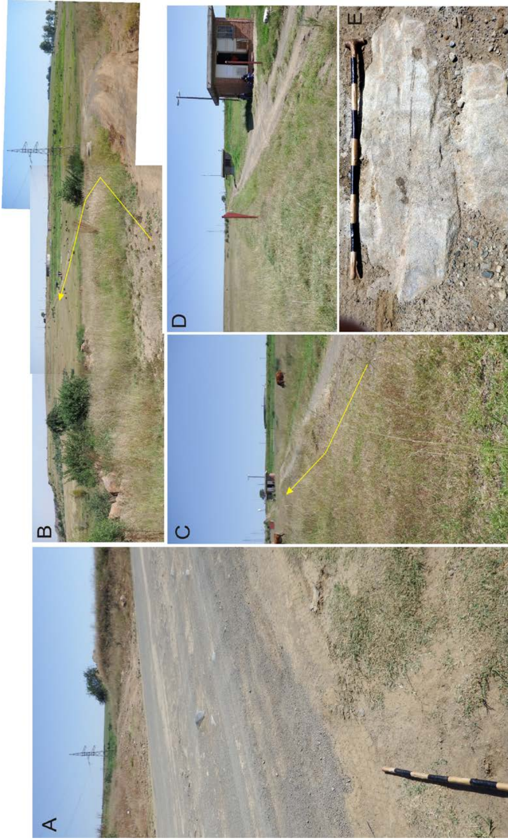
Figure 7. The pipeline crosses J.J. Hadebe Street (A) and then follows the Namahadi WTW access road (B - D) to its termination point at the western boundary of the facility, all underlain by coarse-grained sandstone bedrock (E). Scale 1 = 10 cm.
