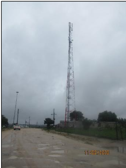
Figure 19 – Communication towers found in the project area
