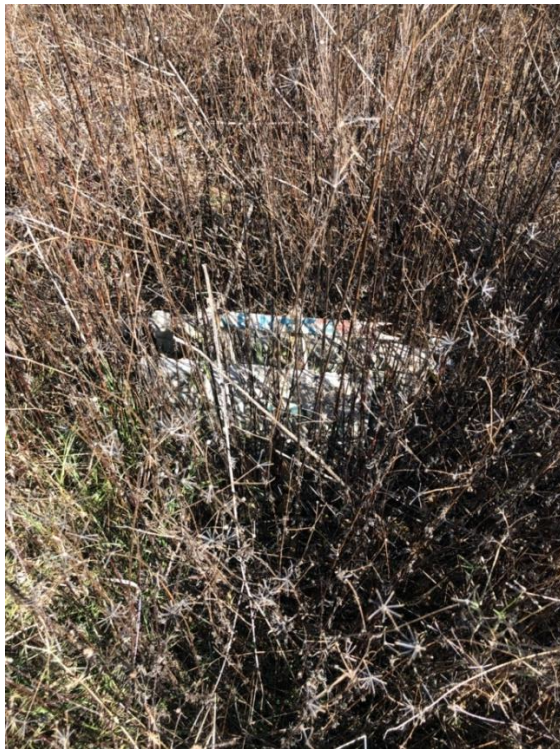
Figure 24 – View of heavily overgrown structure
