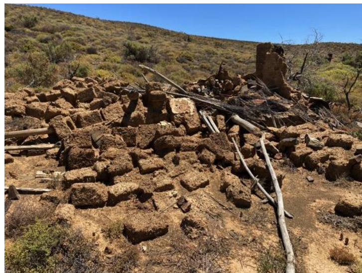
Figure 41: Collapsed mud and grass structure at Stinkfontein
