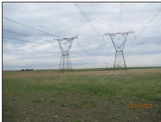
Figure 7 - Eskom Powerlines located on the western section of the pipeline.
