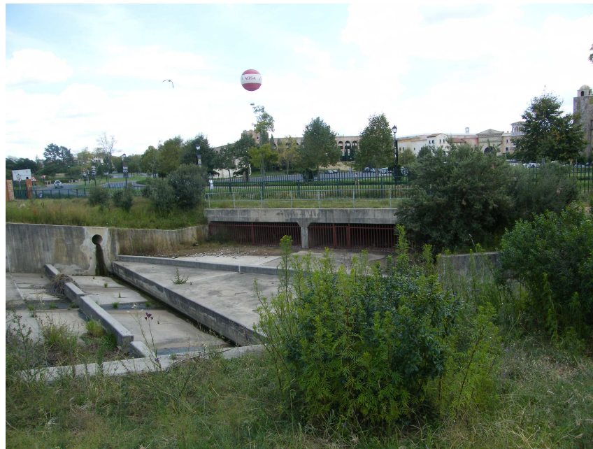
Figure 6: The stormwater control weir located at the outflow of the wetland
