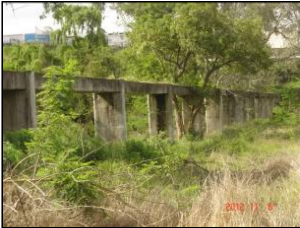
Figure 4 A collapsed bridge (currently not being used)
