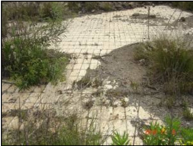
Figure 5 Floor of a collapsed house
