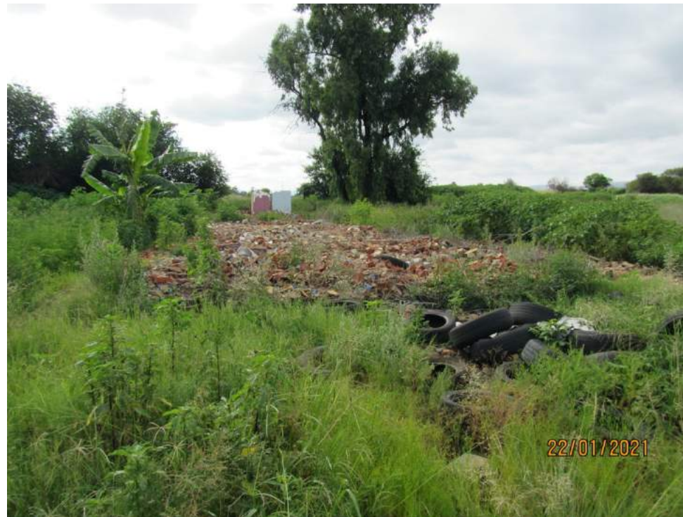
Figure 19 – WK001 View of broken-down structures and piles of building rubble.
