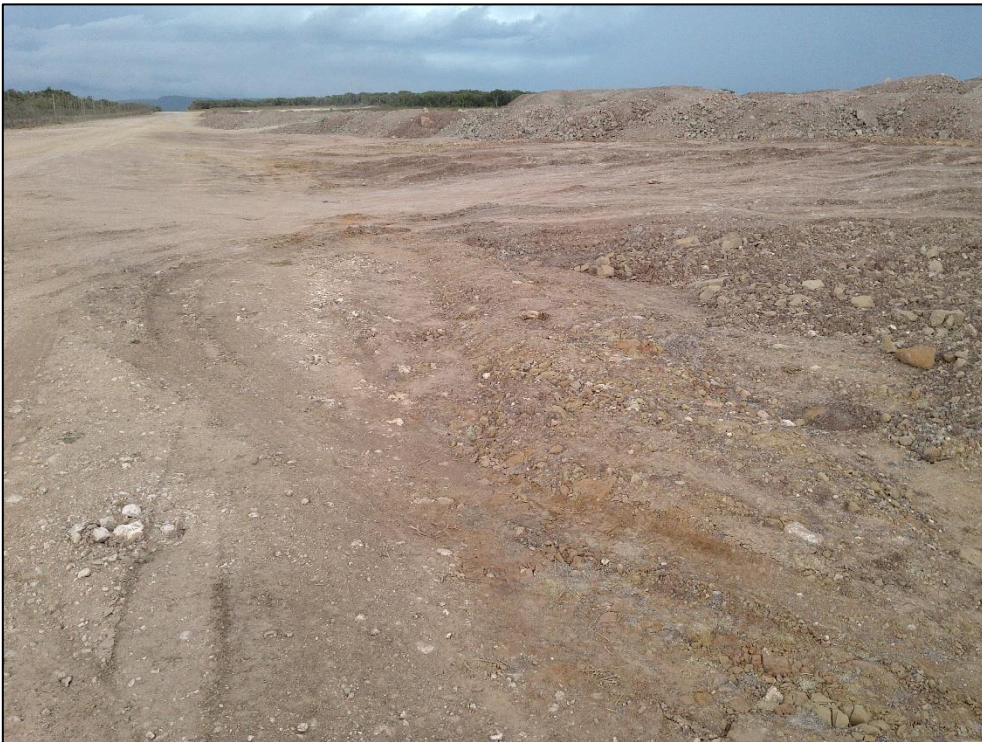
Figure 62. View of the existing borrow pit / mining activity (Existing BP6 [2], Fig 60) situated south of the proposed Borrow Pit 6 (BP6) area.
