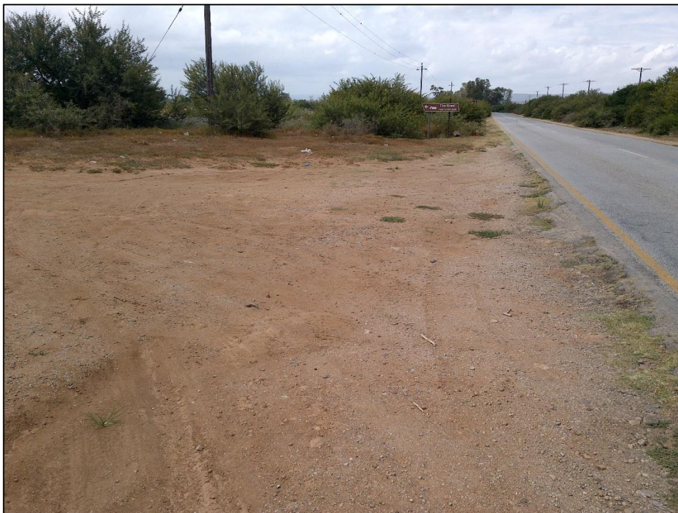
Figure 4. View of the road reserve proposed for upgrade (km 0.5– km 12) facing north towards Addo Town.
