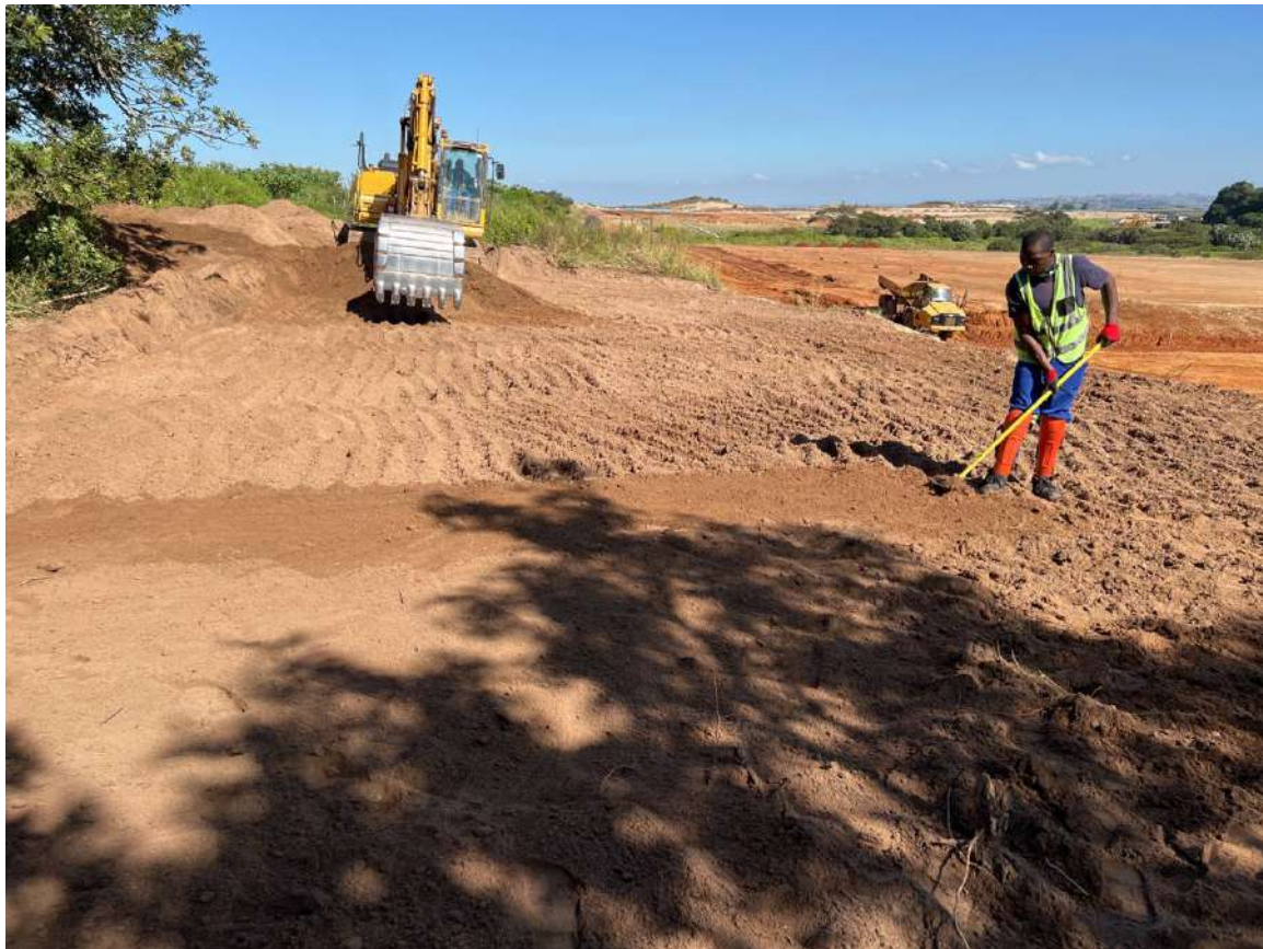
Figure 15 – Further levelling of the site by hand and removal of vegetation remnants
