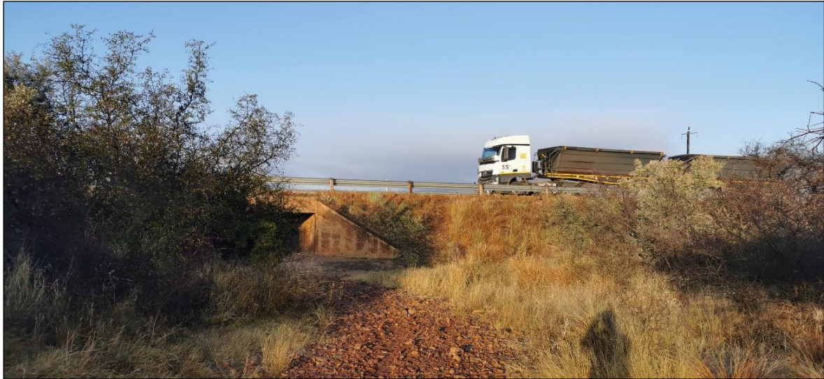
Figure 7 - View of a bridge and the storm water drain located beneath the R31 main road.
