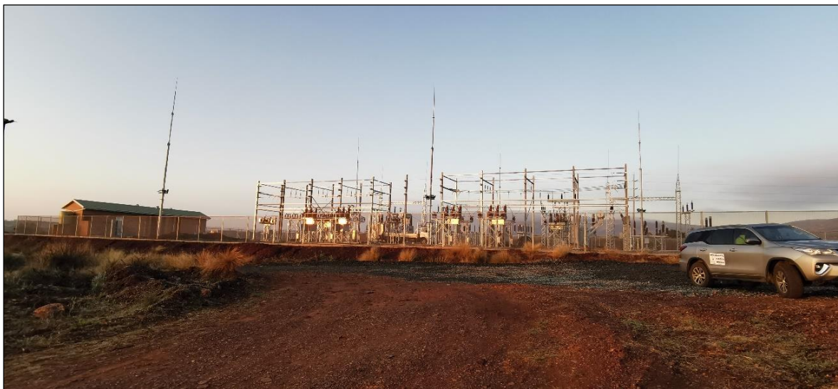
Figure 4 - View of the Gamohaam Substation.
