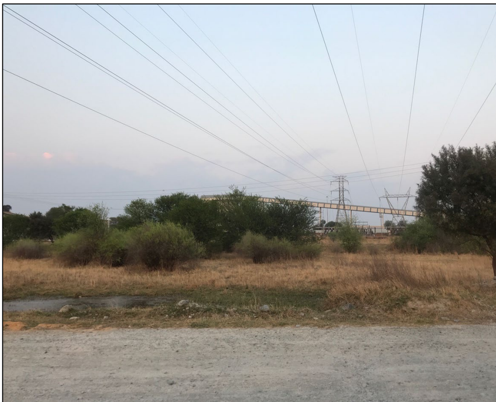
Figure 16: View towards the Vaal Reef ten Substation.
