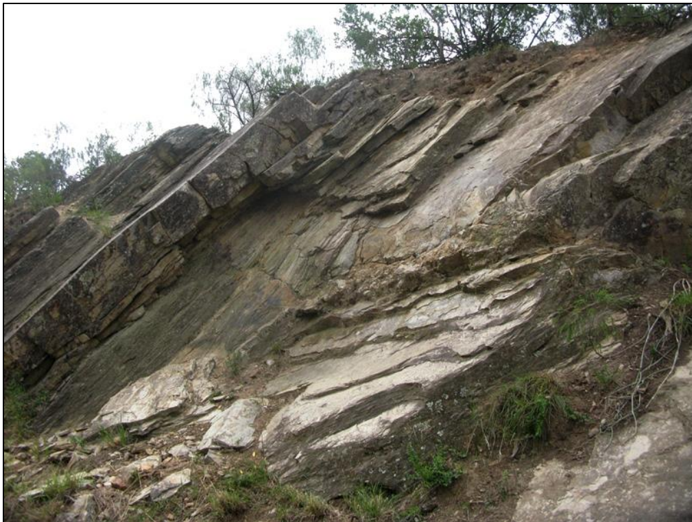
Figure 10. R102 road cutting through folded quartzitic wackes and phyllitic pelites of the Sardinia Bay Formation, c. 1 km west of Van Stadensrivier (Loc. 025). Similar deformed siliciclastic sediments are likely to underlie the grid connection corridor to the NW of Thornhill but are not well exposed there.
